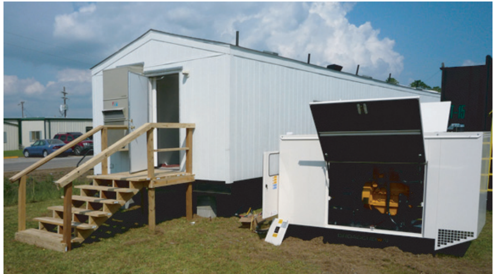
Fully self-contained mobile Shower/Bath building with electric generator and 16,000 gallon water and sewer capacity. This air-conditioned unit provides 13 shower stalls, 8 toilets and 320 gal.s of hot water
